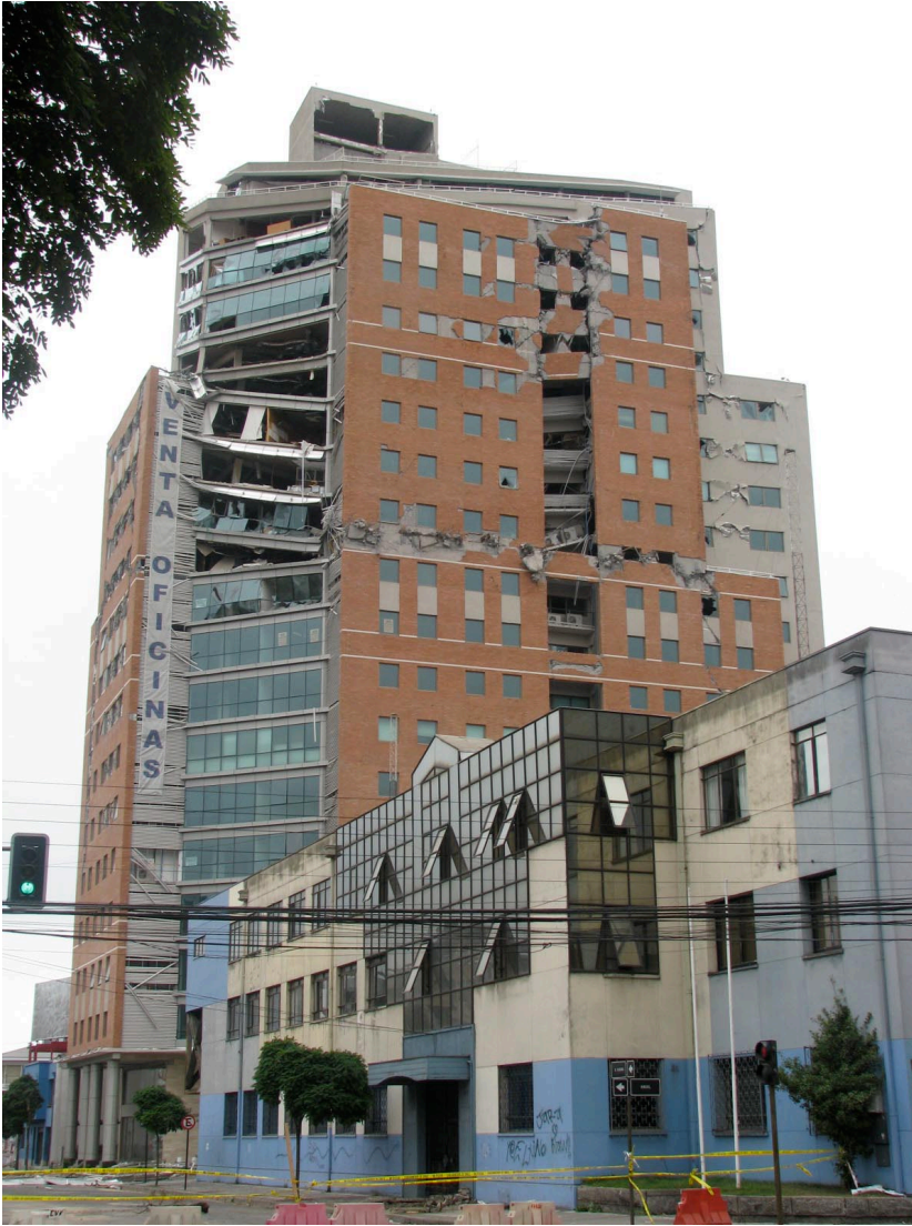
One of the few newer buildings in Concepción with major structural damage. The 11 th floor collapsed. Fortunately the building was unoccupied at the time.
