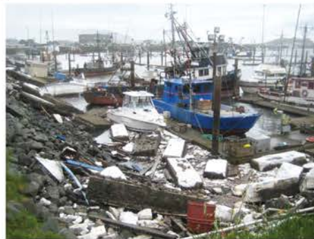
The damage at Crescent City.
