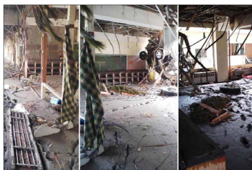
Debris from the tsunami, including a car, litters the third floor of the Kamaishi Junior High School.
